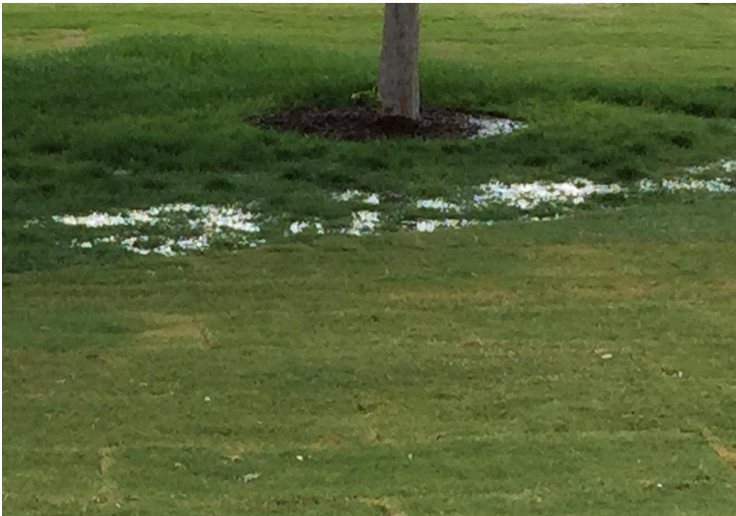
Figure 98: Irrigation zone leak near the Easter Pageant stage area. This leak is especially troublesome because it is in an area of high importance with freshly laid sod.
