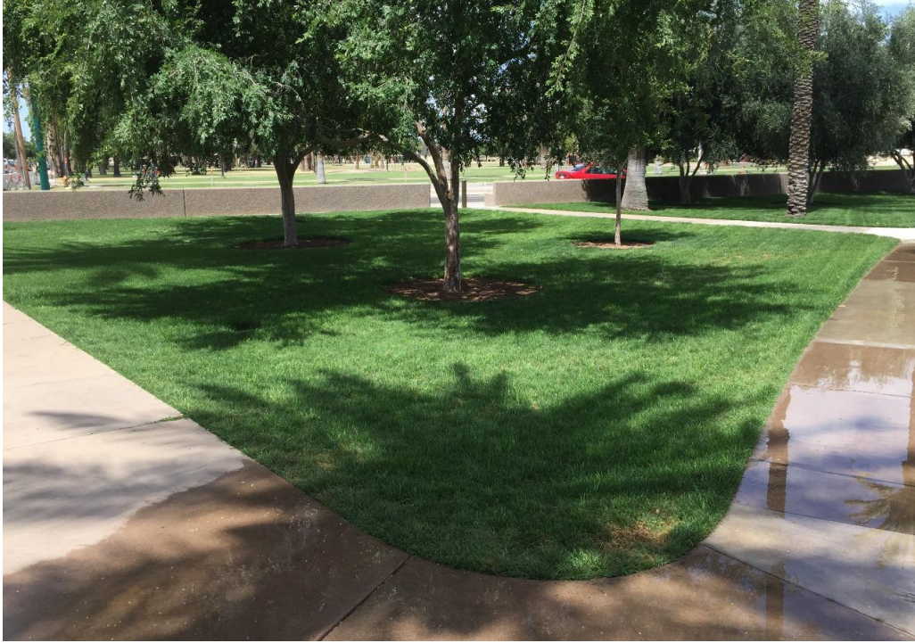
Figure 97: Long term irrigation system leak in the Northwest Lawn of the Mesa Temple grounds. This leak has persisted for the duration of the Vita projects despite multiple discussions with Temple maintenance personnel.
