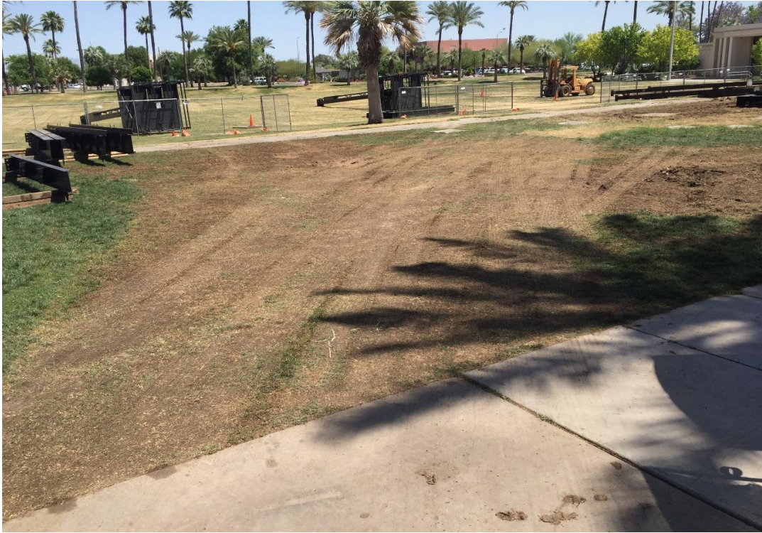
Figure 61: North side of the Easter Pageant stage during disassembly of the stage – 22 April 2015.
