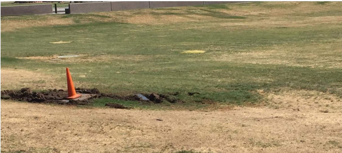
Figure 24: View looking northward around the northwest circumference of the North Mall. Notice the rim of the bowl appears dry while the foot of the slope is greener, a variation caused by the discrepancy in water. The large sum of water pooled in this view is from a leak and further demonstrates the challenges for irrigating sloped terrain.
