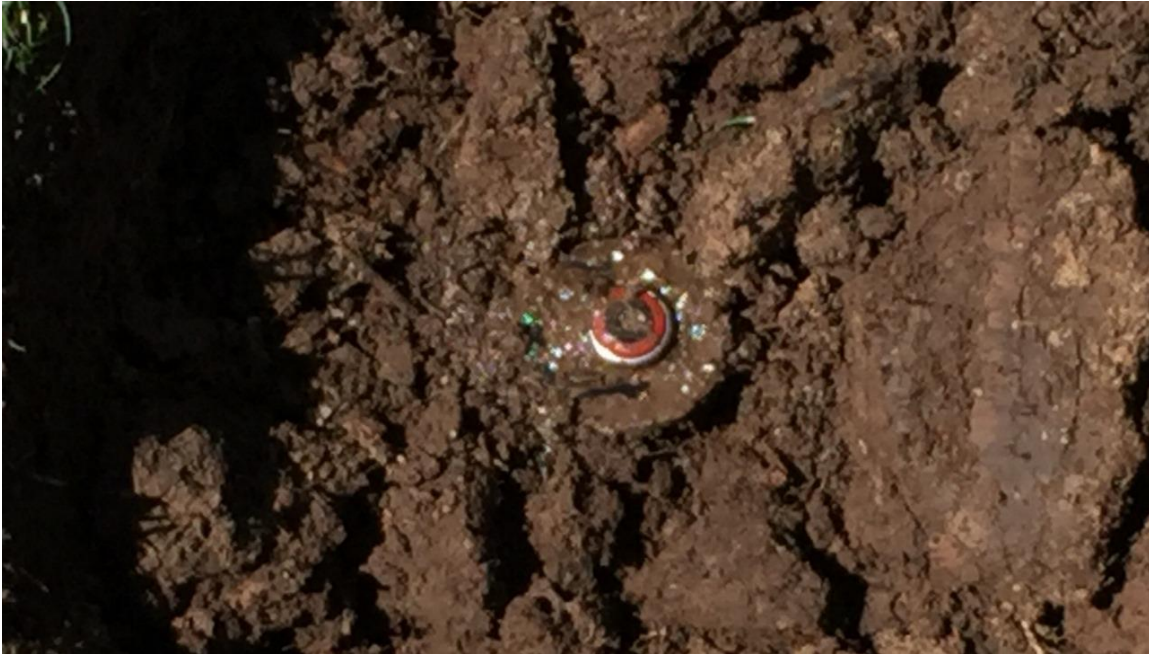
Figure 100: MP Rotator sprinkler head in Zone 84 that was completely buried. This head was found during a sprinkler system audit performed by Growing Season, Inc.
