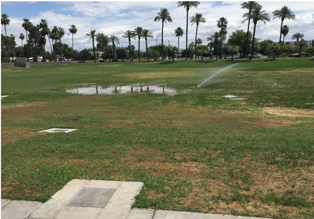
Figure 99: Large irrigation system leak in the North Mall area.
